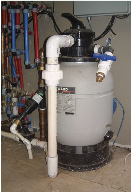
Graywater sand filter at the Sunset San Francisco Idea House. Photo: WaterSprout.
