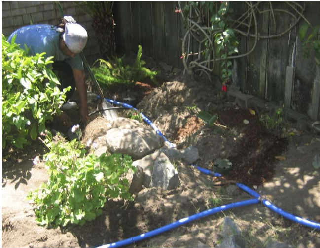
1-inch Blu-lock HDPE tubing laid out in trenches. All tubing was buried after system was finished. Photo: Laura Allen.
