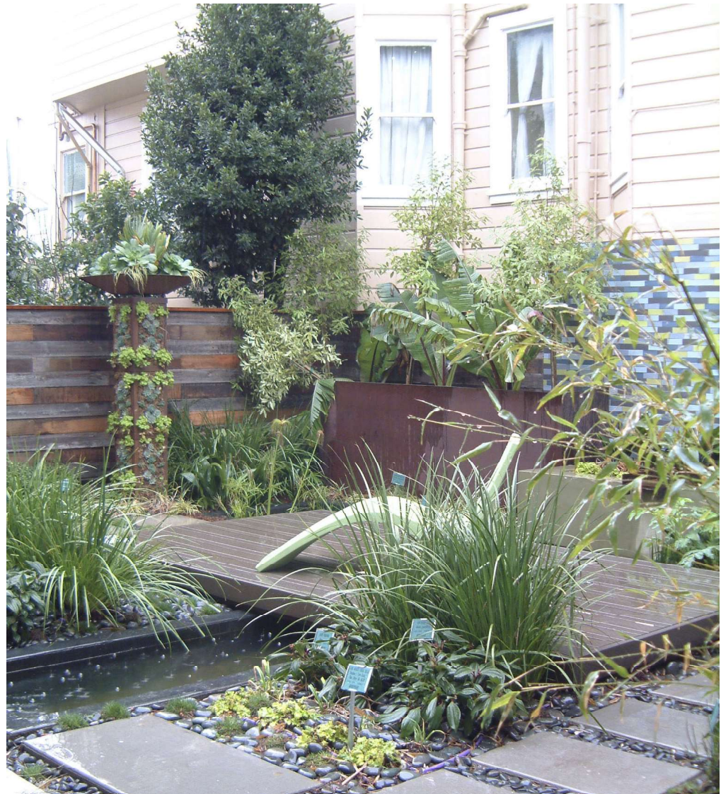
This landscape is irrigated with graywater that has passed through a sand filter before entering the subsurface drip irrigation system. Note: The pond is not supplied by graywater and is lined so that graywater doesn't enter it. Photo: WaterSprout.
