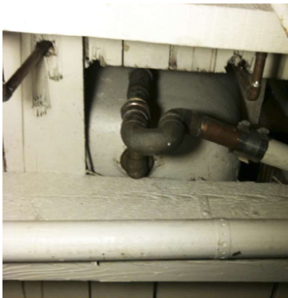
The shower p-trap is the copper pipe shaped like an upsidedown and sideways letter “p.” In this example, the p-trap and shower drainage pipes are located below the shower/tub. Photo: Josh Lowe.
