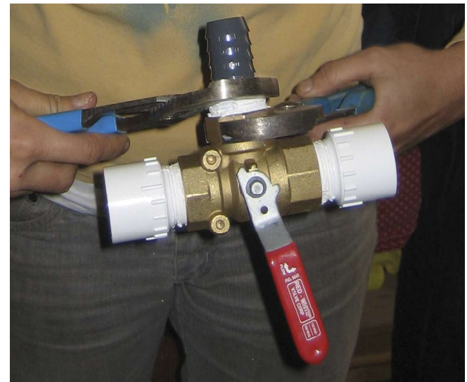
Tightening fittings onto the 3-way valve with channel locks. Photo: Laura Allen.
