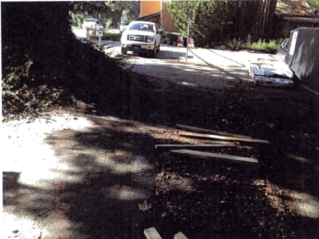
Root system and root flare lifting the parking area
