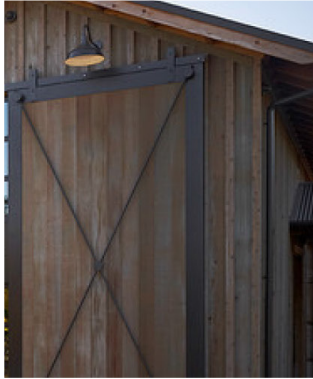
VERTICAL WOOD SIDING: Board & Batten w/ full 2"x4" battens. Western Red Cedar (STK) w/ a portland cement wash treatment (to age) and a clear coat over that
