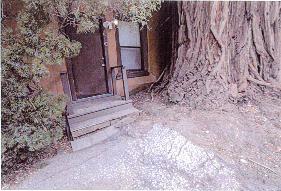
Example of damage at east facade (Architectural Resources Group, March 2016)
