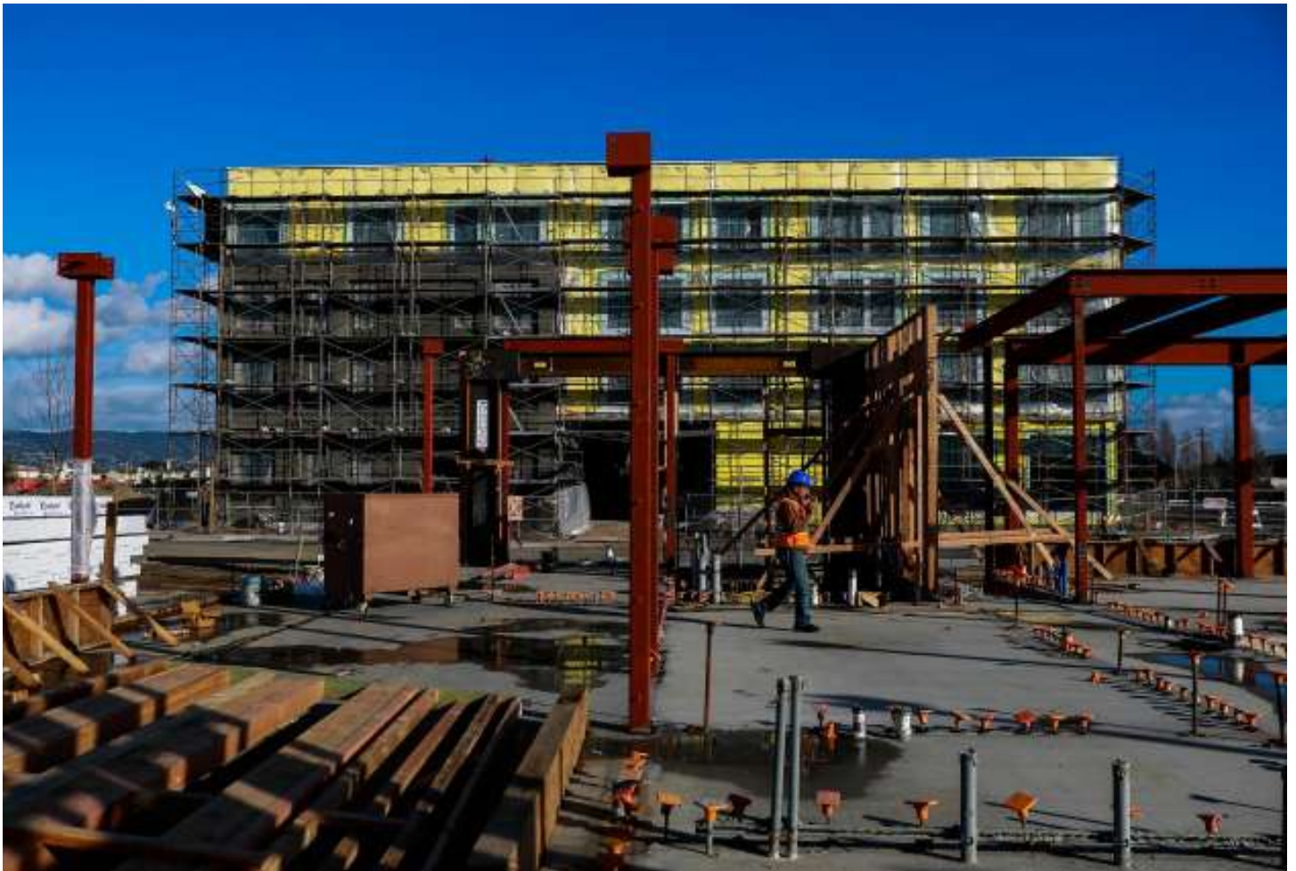
A construction worker walks past the site of a new condo under construction site at Alameda Point on Tuesday, Jan. 14, 2020 in Alameda, California.
