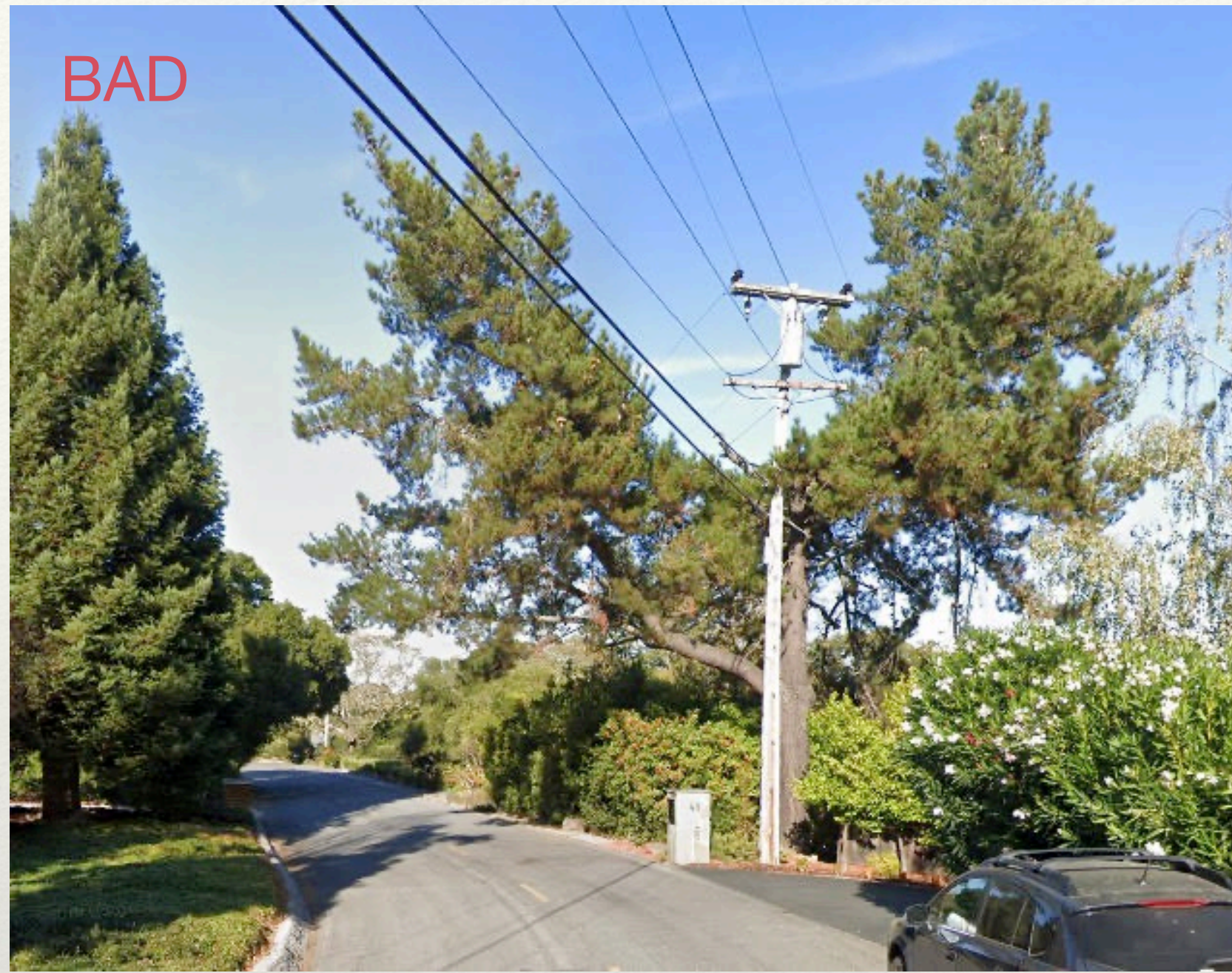
Overhanging Pine in Right of Way
