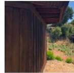
Existing Rusted redwood sidings
