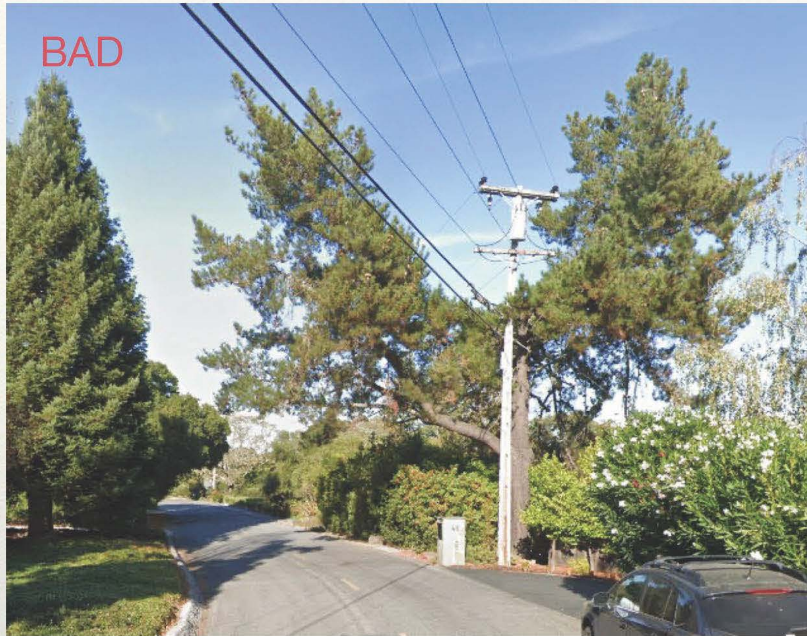
Overhanging Pine in Right of Way
