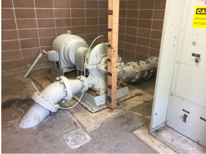
Photo 1) Photo inside of the building showing old out of date booster pump and 4x4 wood post roof support.
