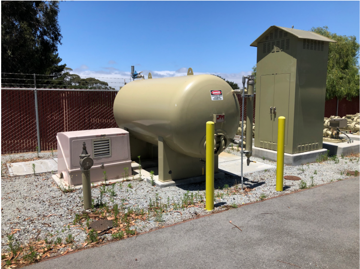
Photo #7) Photo of hypopneumatic tank and acoustical shelter for reference. Similar concept
