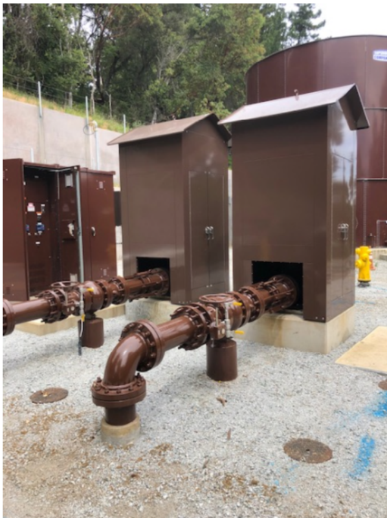
Photo 6) Example of outdoor acoustical shelter and pumps at another station in Bear Gulch. Colors to match or as approved by Portola Valley. Station piping shall look the same and shall be similar. Height of acoustical shelter will vary but will be fairly close to matching this example.
