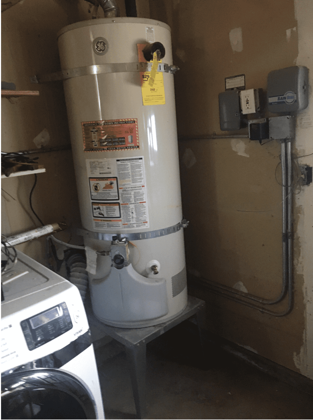
Today: 50-gallon gas tank WH in garage
