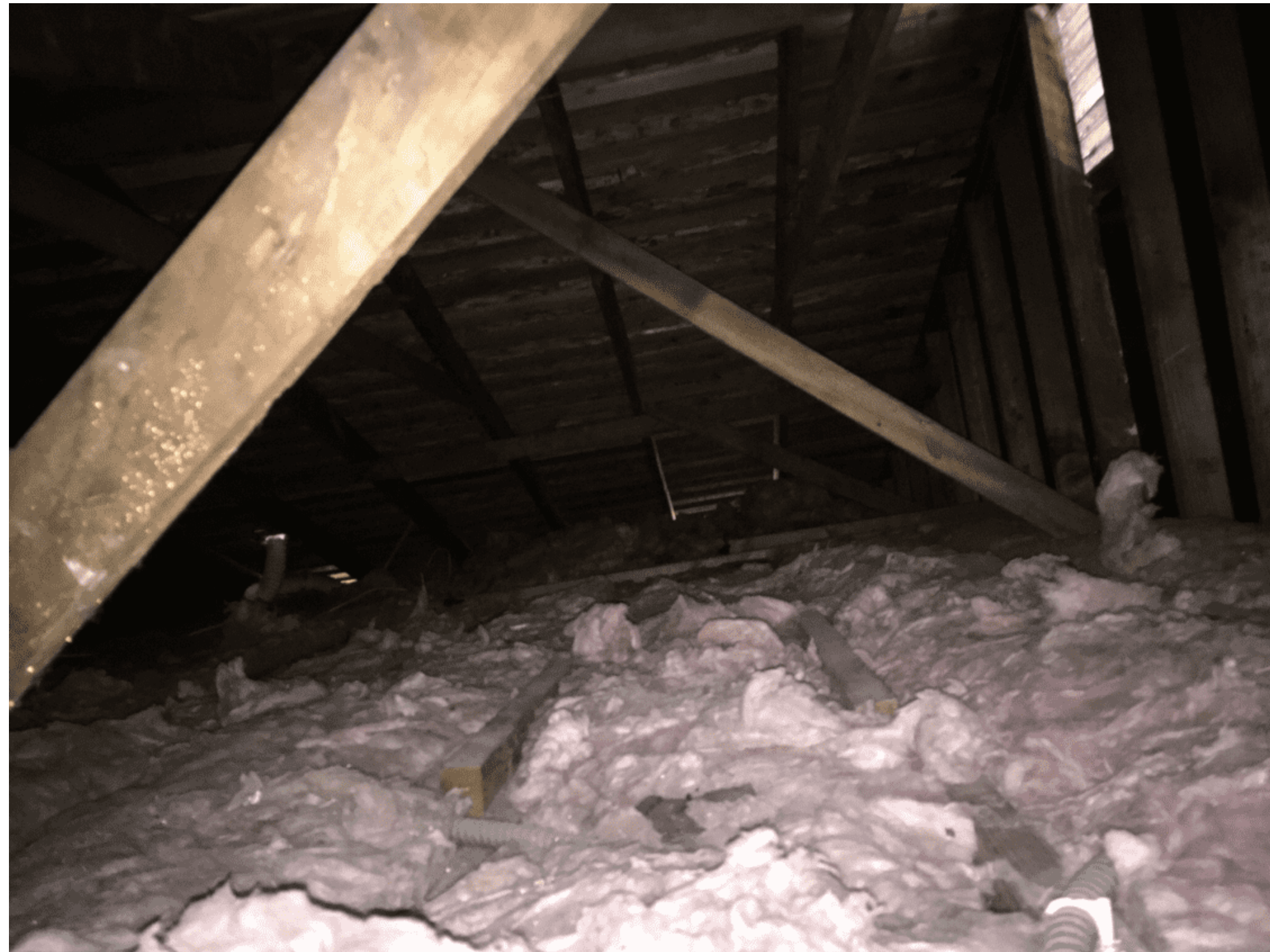
Today: Attic, R-19 insulation Recommend: R-38
