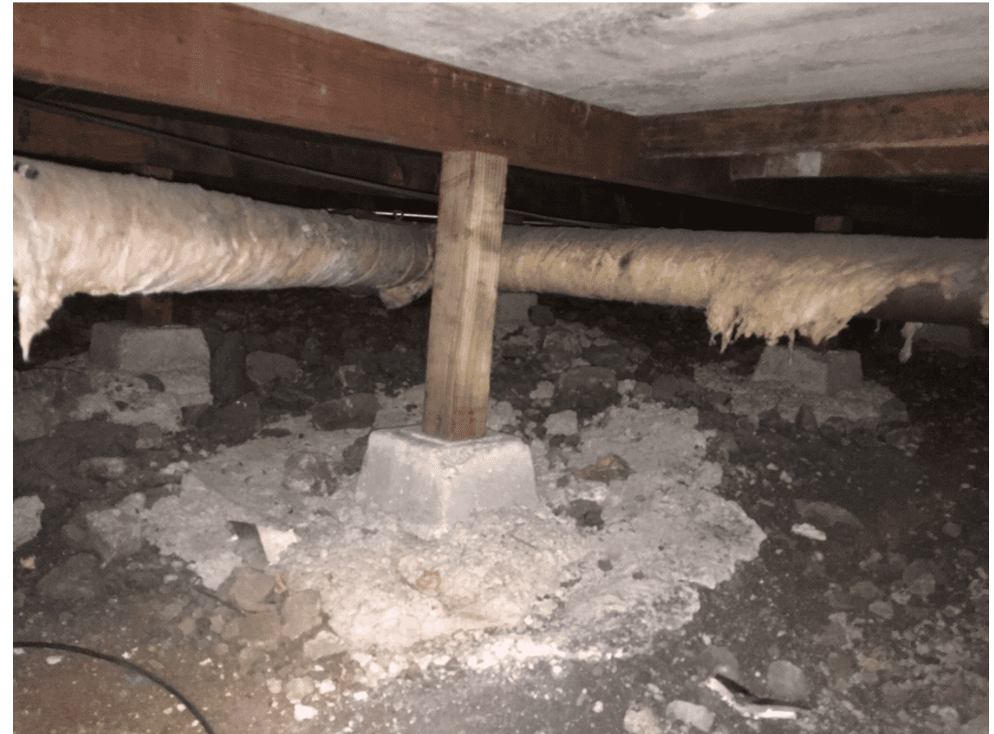
Today: Crawlspace, no insulation, poorly insulated ducts Recommend: R-19 or R-30 for floors, repair ducts
