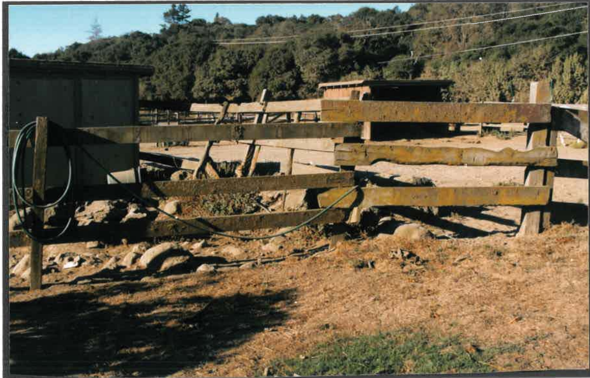
Photo 3. Chewed and rotten boards and posts were evident everywhere
