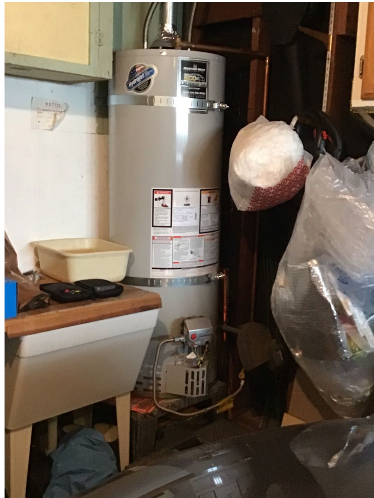
Today: 50-gallon gas WH in garage
