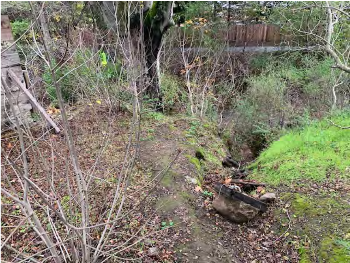
Photograph 2 – Erosion gully west of the beer garden fence (photo left) that accepts large amounts of runoff from the unpaved parking area. Roots of the large oak are being exposed in the gully.
