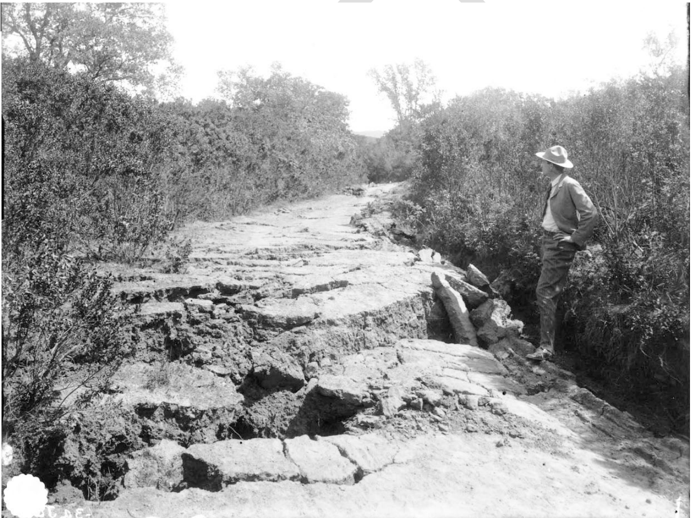
Vertical offset of Alpine Road 5 miles west of Stanford University. Per J. C. Branner. 1906 photograph from The California Earthquake of April 18, 1906: Report of the State Earthquake Investigation Commission (1908).
