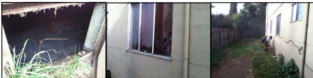
Left to right: stagnant water under a building in San Mateo; condensation on window; and Richard Chow using a backpack fogger to apply an adulticide treatment underneath the building.
