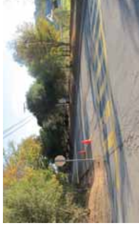
Faded lane, crosswalk, and stencil markings at Alpine / Corte Madera.
