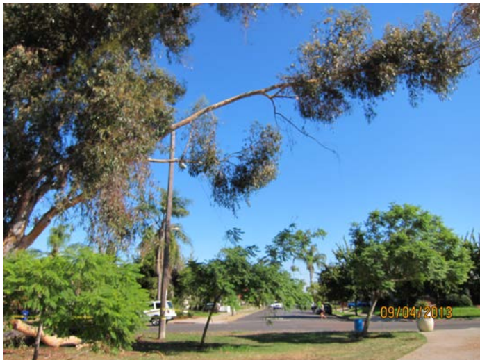
A limb extended over a pedestrian sidewalk from a tree with a previous history of failure is a red flag warning for removal
